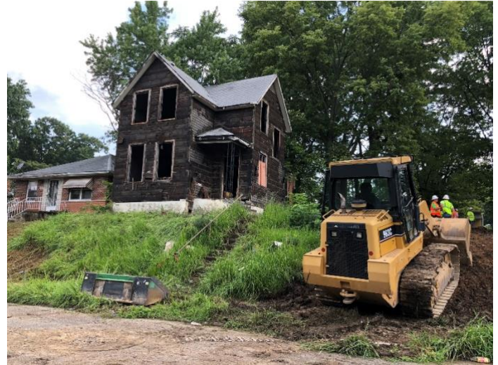
Construction and contractor crews donated their time and equipment to take down vacant houses, including this house in the 27th Ward.
